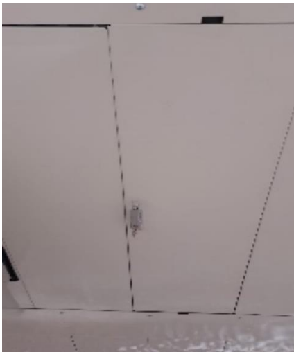
Fig.1 Panel locked with key
